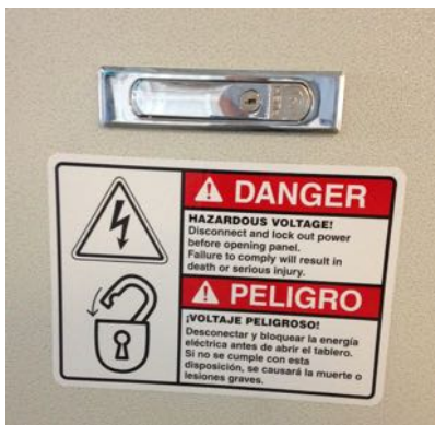
Figure 8-2 - Electrical Panel Door Lock
