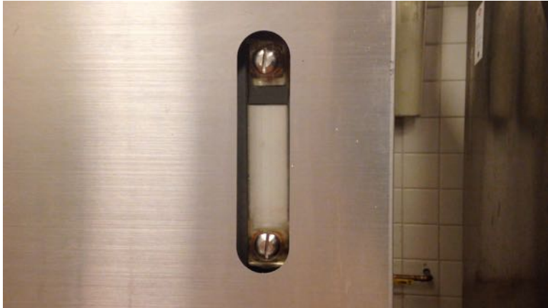
Figure 8.6 – Deodorizer Level Gauge
