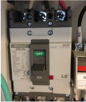
Figure 8-3 - Digester's main breaker switch (in the OFF position)
